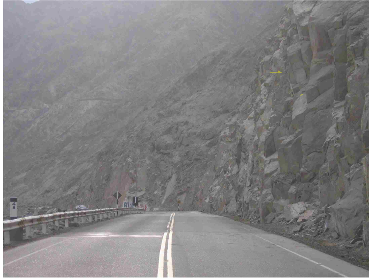
(a) Blocky slope with indications of missing rock blocks where toppling and slumping failure modes are suspected.
